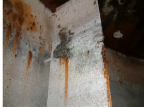
Photo 8 ** Deteriorated Baffle Limestone Slurry Tank
