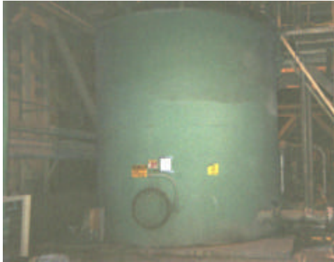
Photo 7 FGD System Bleed Tank
