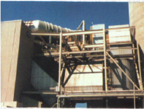
Photo 3 Scrubber Bypass Duct
