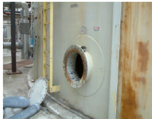
Photo 10 ** Exterior Corrosion on Slurry Feed Tank
