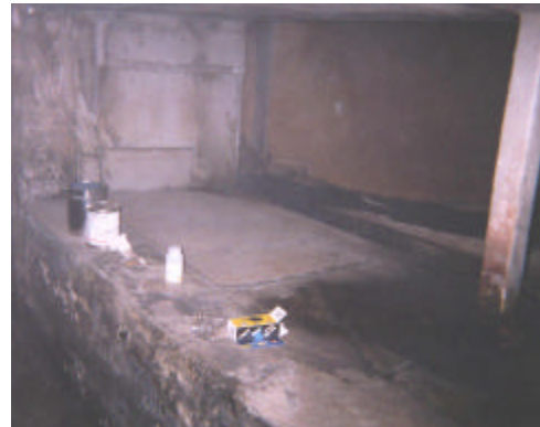
Photo 4 Scrubber Inlet Duct
