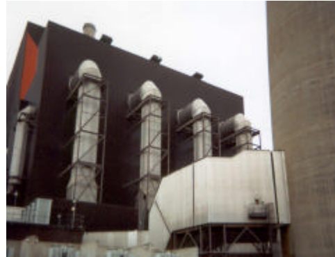
Photo 2 FGD Outlet Ducts and Breaching
