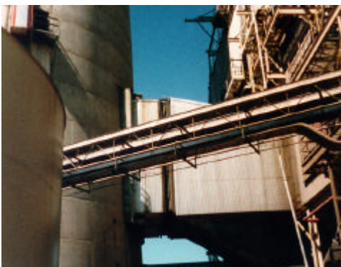
Photo 5 Precipitator Outlet Duct/Breeching
