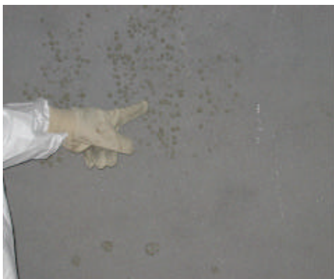
Photo 9 ** Severely Pitted Tank Interior
